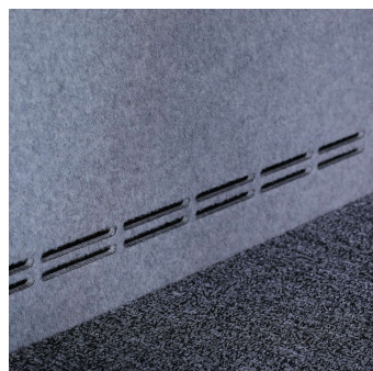
Air outlet near the floor
